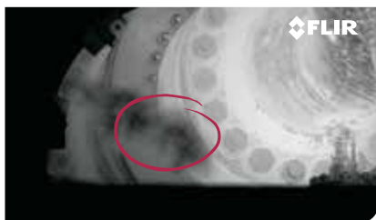
A leaking flange.
